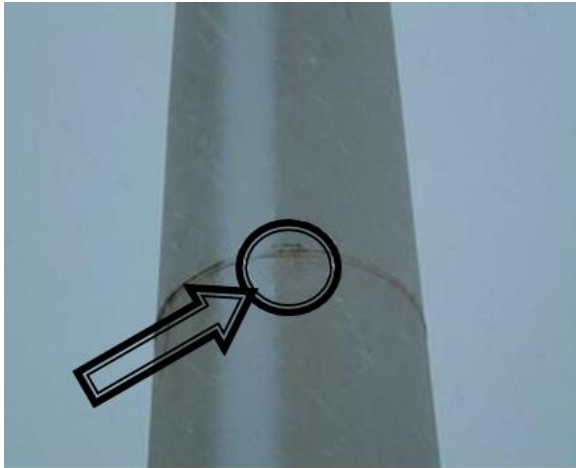
Crack in the weld of the tower
